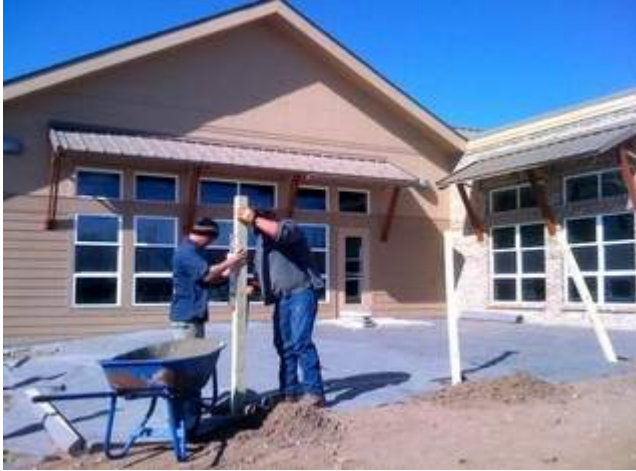
Jesse Martens and Delmus Garber install fence posts outside the nearly completed Sister Mary Alice Center for Hope in Fort Collins. The fence will enclose a childrens' play area. (Coloradoan/Trevor Hughes)
